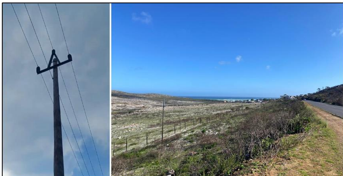
Figure 14. The electricity line that runs between Kogelfontein and Scarborough.
